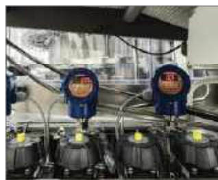
01 Pressure Gauge & Control Valve
