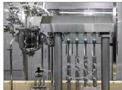
03 Service tank & Pump station
